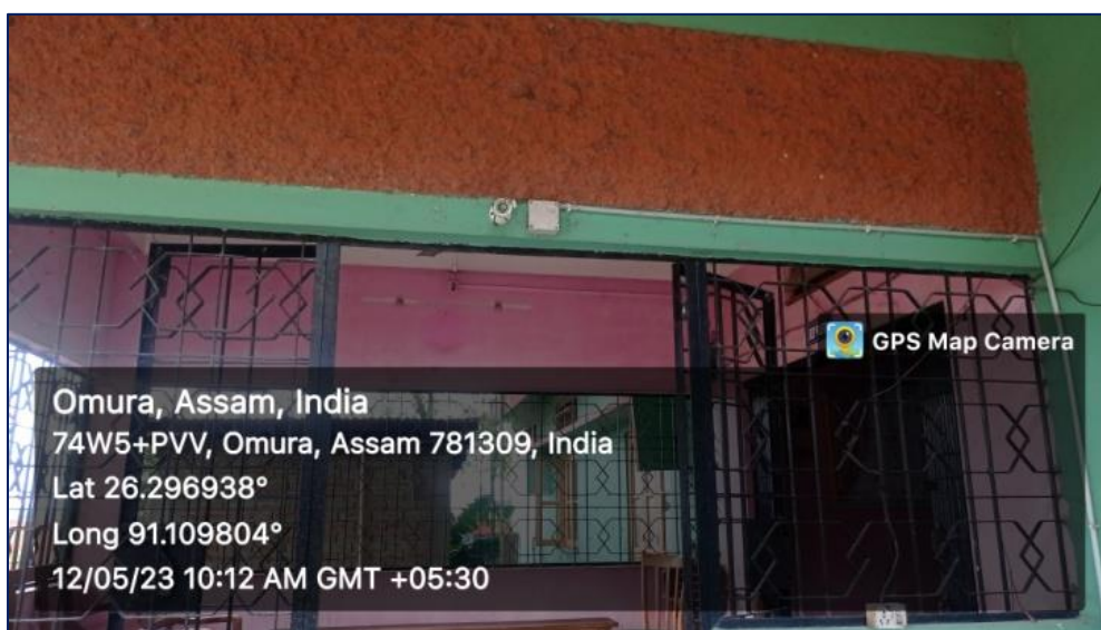
Fig: CCTV installed in Women's Hostel for security to the inmates
